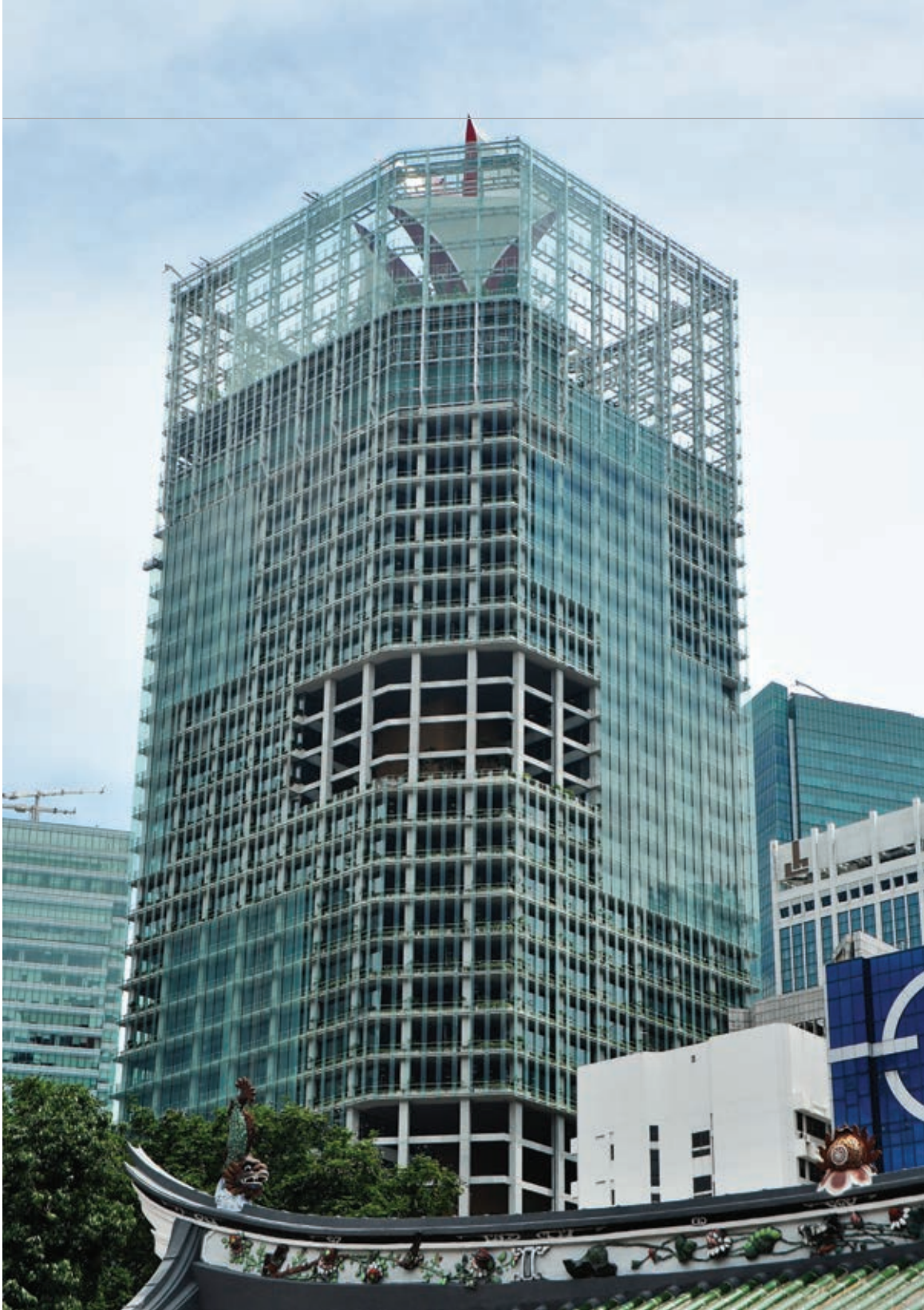
Left: The 40-storey CapitaGreen building under construction in Singapore. Photo: M Metal Pte Ltd.
