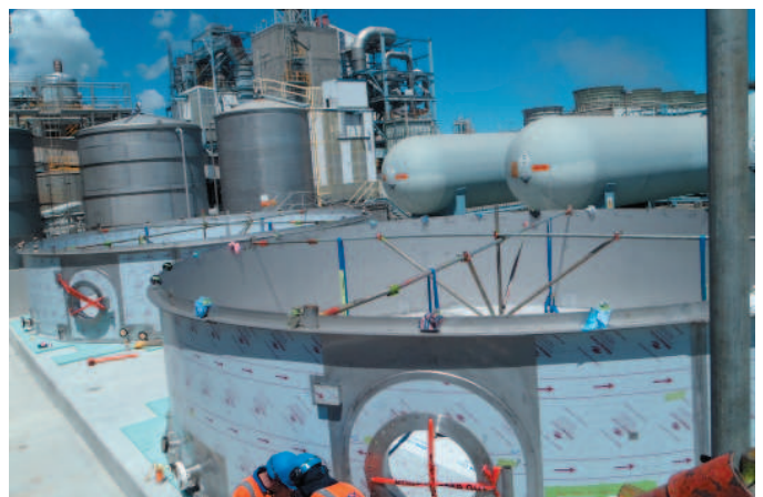
Stainless steel tanks designed and built by HERA member Fitzroy Group delivered in halves and then welded on-site at Ballance AgriNutrients, Kapuni
