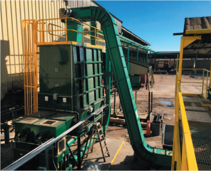
Export success from HERA member Windsor NZ who designed and fabricated five biomass fuel transfer systems installed in the USA earlier this year
