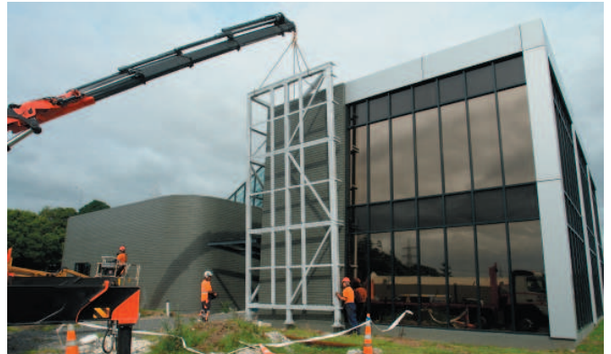
HERA House metal facade frame built and installed by HERA member ISSA Engineering
