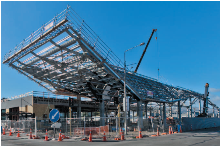
HERA member D&H Steel Construction fabricated the steelwork for the new Christchurch bus exchange
