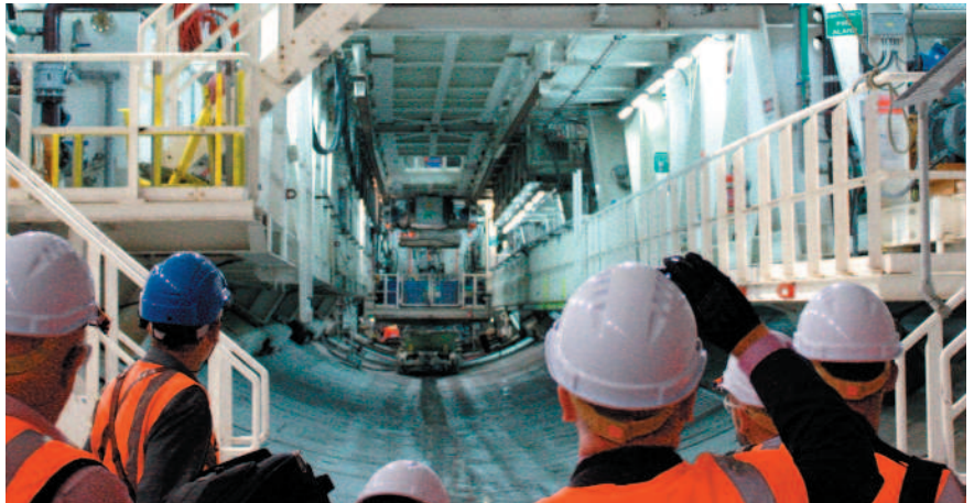
Media tour of the Waterview Tunnel being constructed by a consortium including HERA members Fletcher Construction, McConnell Dowell Constructors, Beca Infrastructure and Tonkin & Taylor
