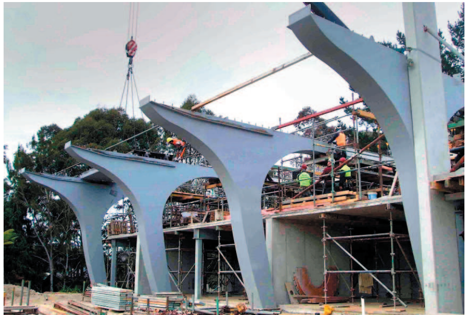
HERA member Jensen Steel fabricated the steelwork for the award-winning Ratcliffe Riverhouse in Hamilton designed by HERA member Holmes Consulting Group
